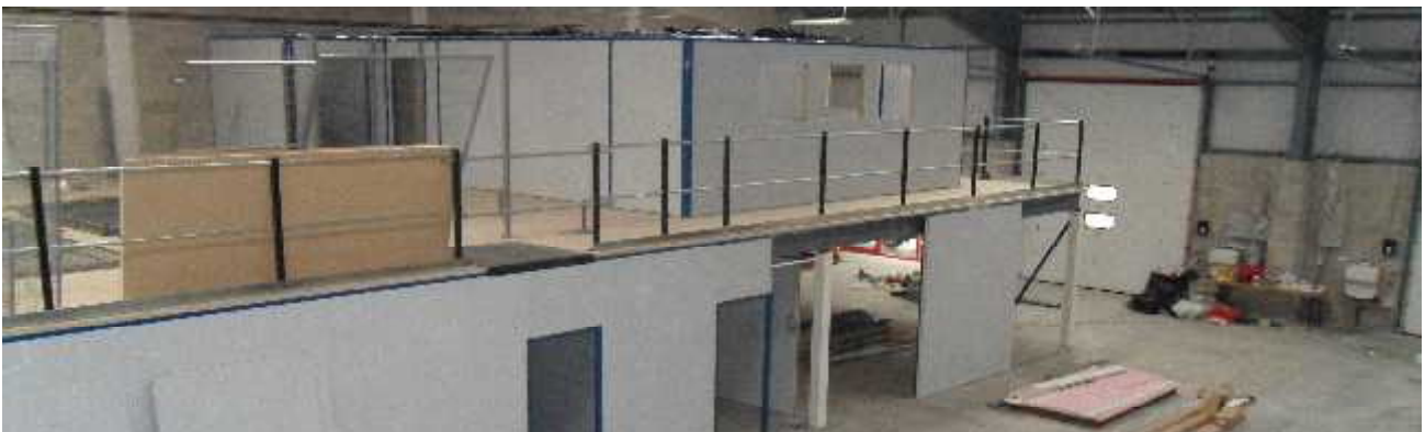
A 'mezzanine' industrial partitioning system in mid-build, demonstrating the joint expertise of Dave and Eric
